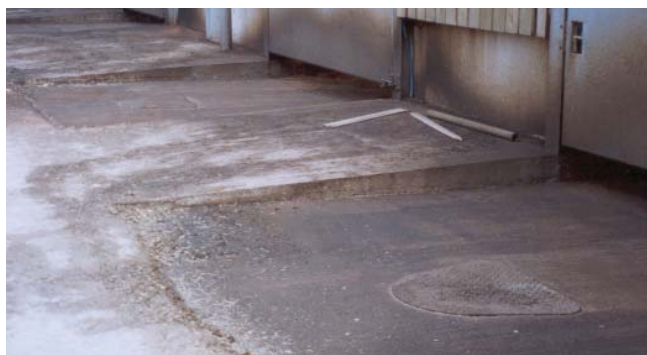
Flush wash valve placed outside a building, centred on a feed passage. Unfortunately the flush wash is hampered by the external gates as shown by the slurry deposits
