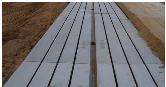
Installation of a slotted drained floor on a sand base. This will form an access pass between cubicles.
