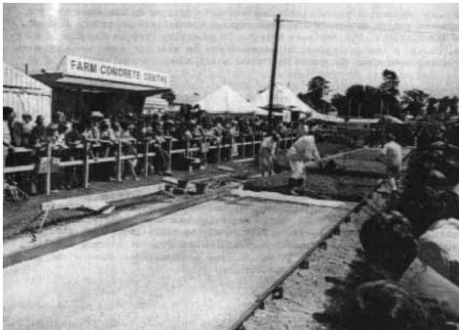
A well attended practical demonstration organised by Maurice Barnes, a Council Member, Cement and Concrete Association.
