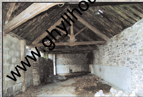
Top: holiday unit barn prior to conversion. Above: inside of barn prior to conversion.
